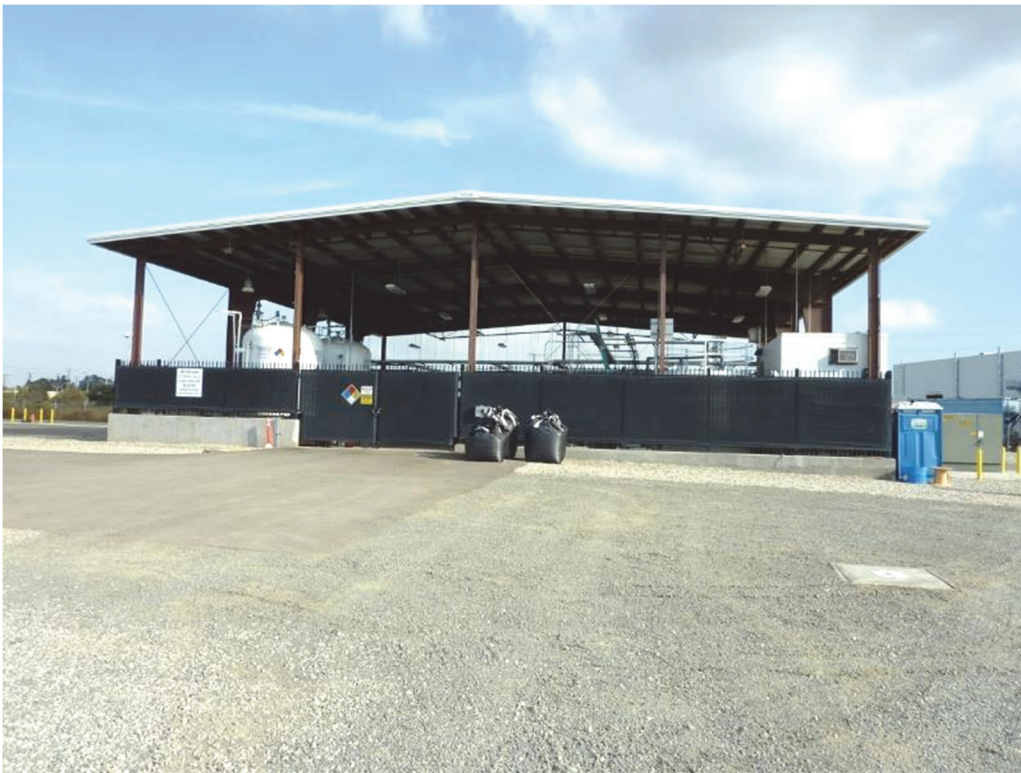
J-5. Groundwater amendment building, part of ongoing EISB effort, in southwest corner of site (11/18/2013).
